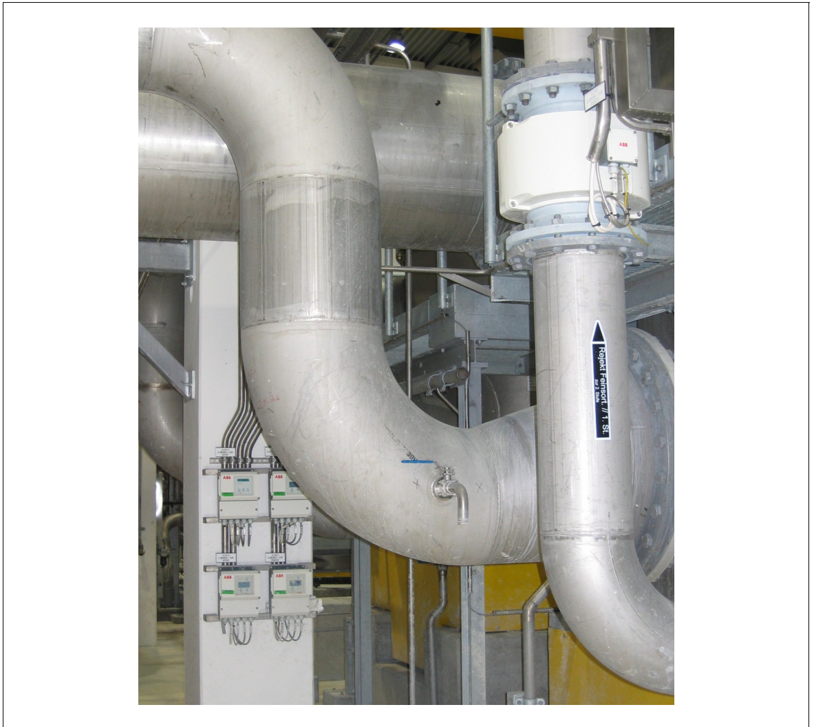
Fig. 1-1: Electromagnetic flowmeter in stock preparation
